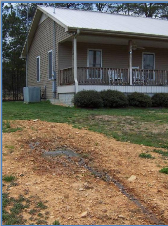
Figure 4.1.c. A failing septic system can introduce pathogens into nearby streams. This system has effluent surfacing in the yard, and drains into a nearby tributary.
