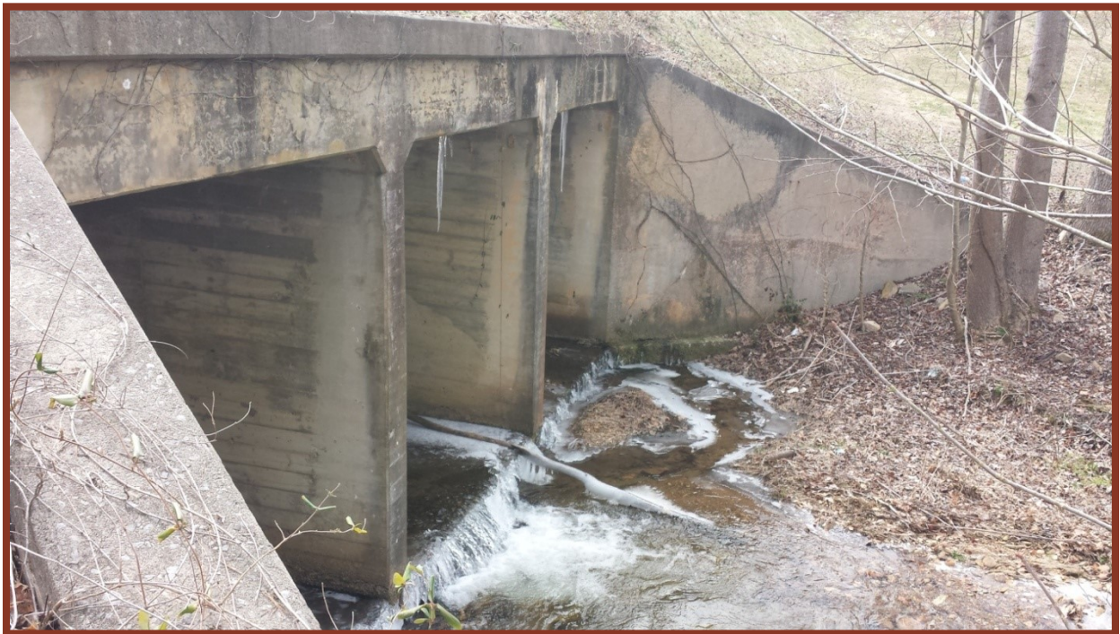
Figure 3.3.g. The concrete box culvert on Holly Creek-Cool Springs Road above Goldmine Branch/Rock Creek.
