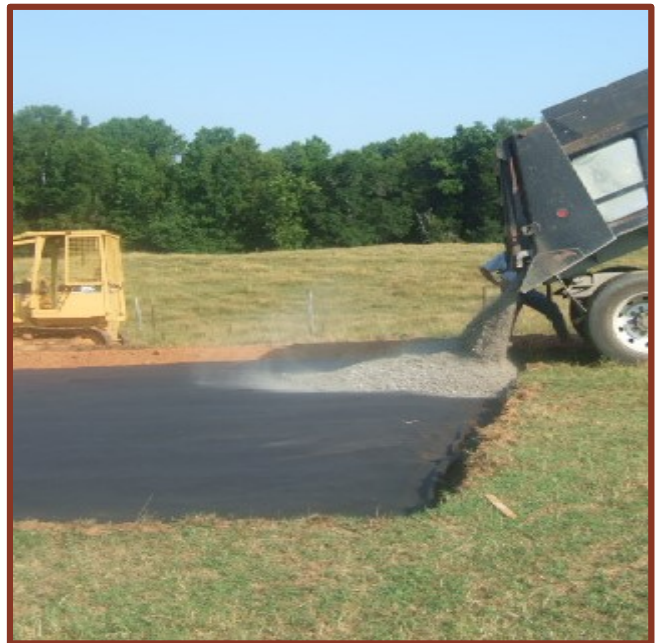
Figure 6.2.a. Constructing heavy use area pads for cattle feeding or watering areas can reduce erosion and sediment loads in the watershed.
