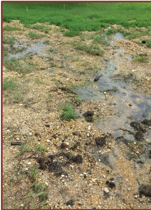
Figure 4.1.g. A failing septic system can introduce pathogens into nearby streams. This system has effluent surfacing in the yard, and drains into a nearby tributary.
