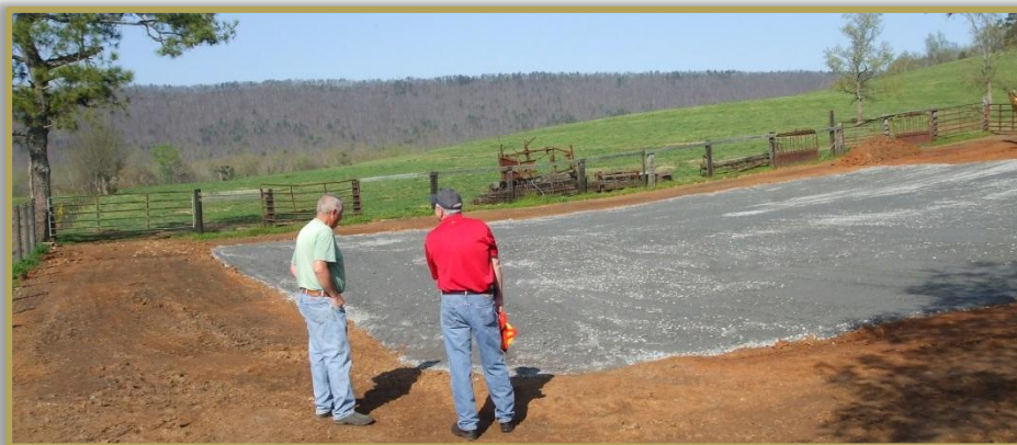
Figure 6.2.a. Constructing heavy use area pads for cattle feeding or watering areas can reduce erosion and sediment loads in the watershed.
