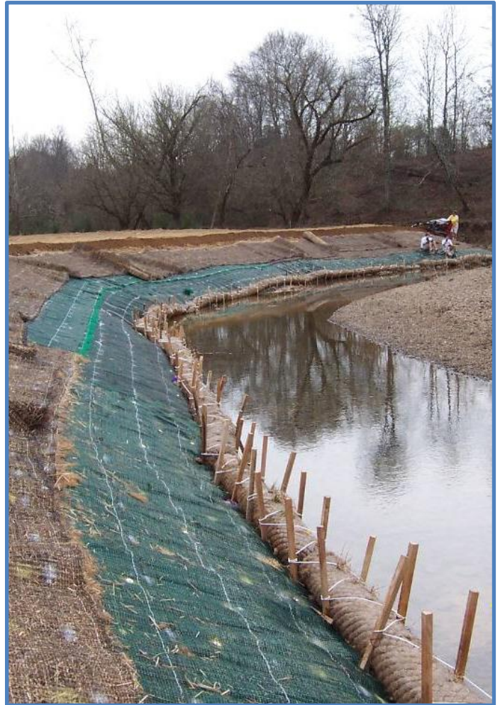
Figure 5.1.a. Streambank stabilization is an important restoration technique where eroding banks contribute to the stream's sediment load.
